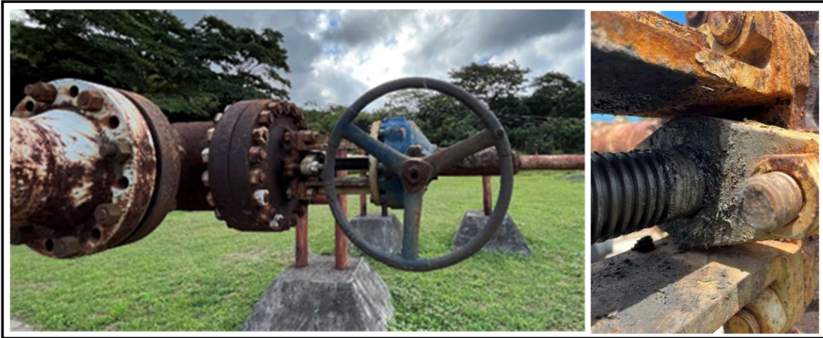
Figure 5: 10" TV in the initial Condition (Left). View on top of packing gland where leak was emanating (Right).
