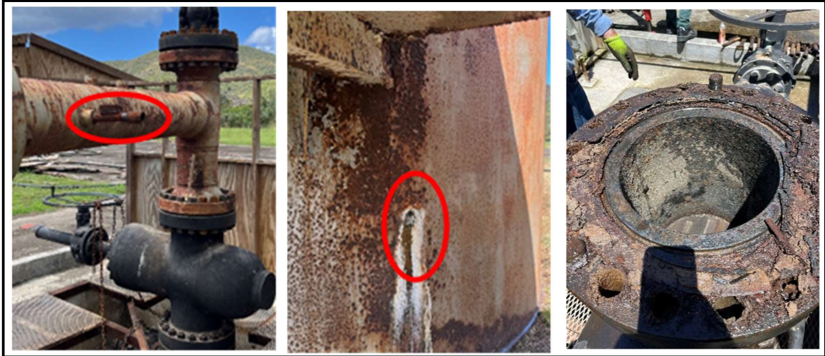
Figure 10: Tap point to be re-worked (Left), hole in separator requiring repair (centre), excessive corrosion on MON-2 12" master valve upper flange face (right).
