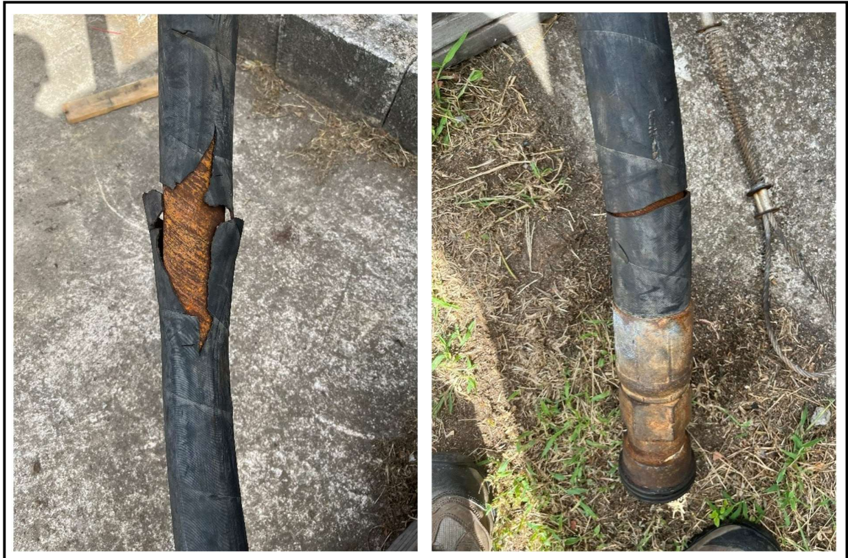
Figure 9: Picture shows the visible signs of degradation of the 2x 2" 250 bar Semperit hoses.
