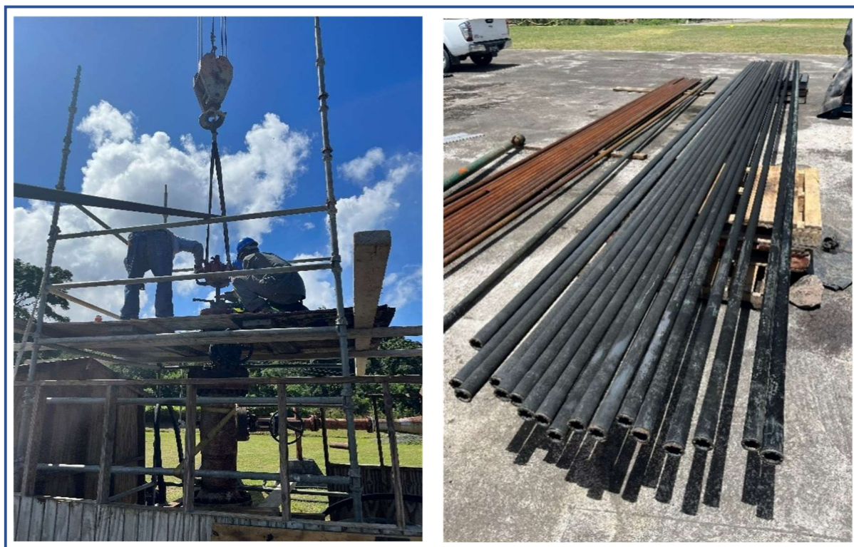
Figure 11: Above shows elevated working platform (left) and pipe rack full of recovered pipe after flowing MON-1 well (Right).
